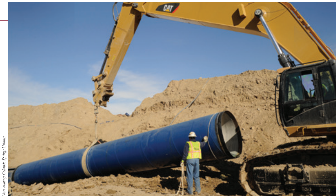
Workers with Garney Construction install a 50 ft., 66-in. diameter pipe segment in SDS
